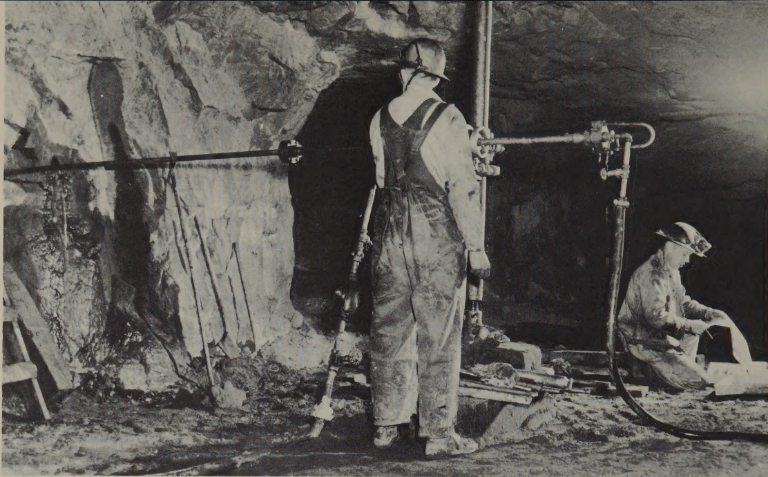
Bureau of Mines engineers conduct a roof-control study at a uranium mine in McKinley County, N. Mex.
